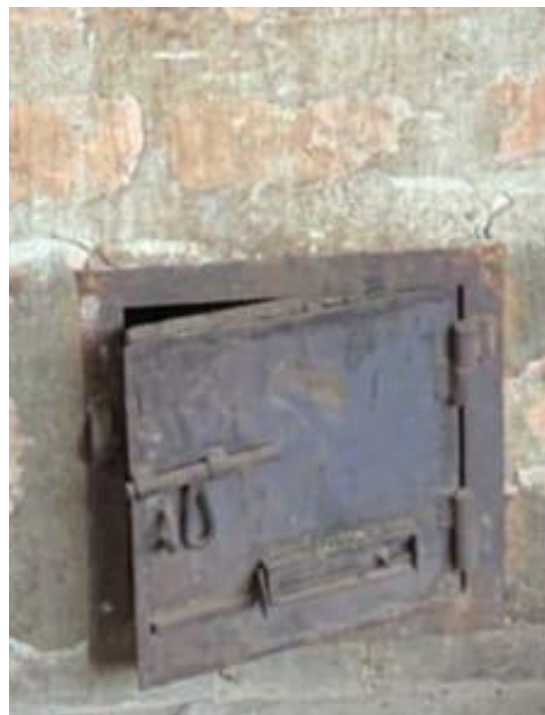
Figure 16: Fire chamber door with air valve and locks
