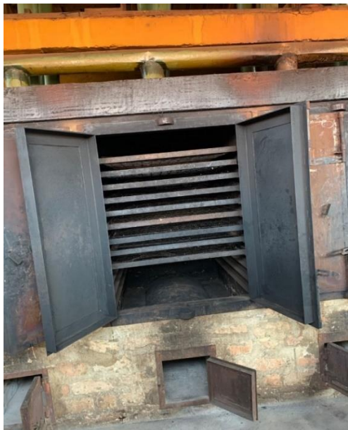
Figure 30: Racks in the oven
