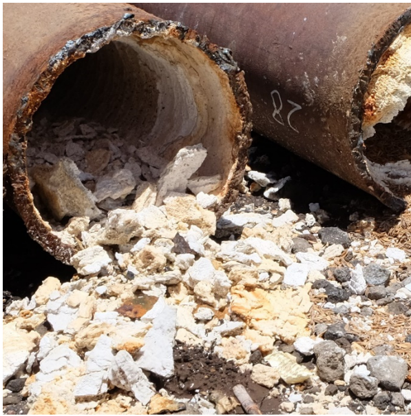
FIGURE 2: Silica scaling at brine line piping
